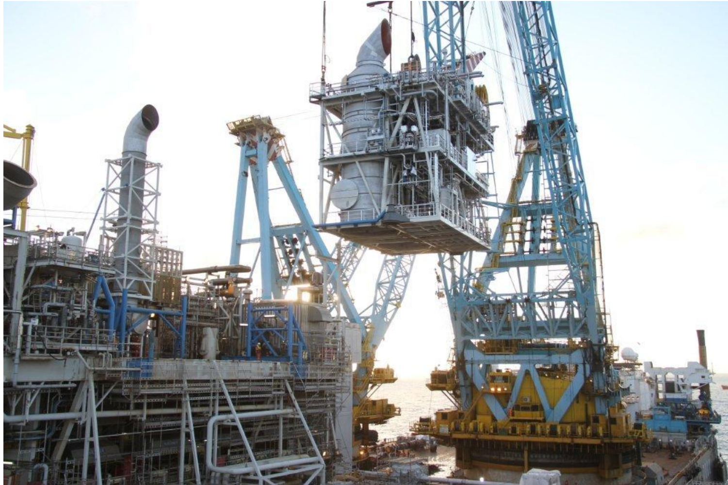
CONOCO PHILLIPS CSG INSTALLATION - ELDFISK PLATFORM
